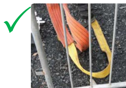
Additional protection added to protect sling from damage (sharp edges)!
