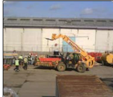
Attachment and load incorrectly positioned
